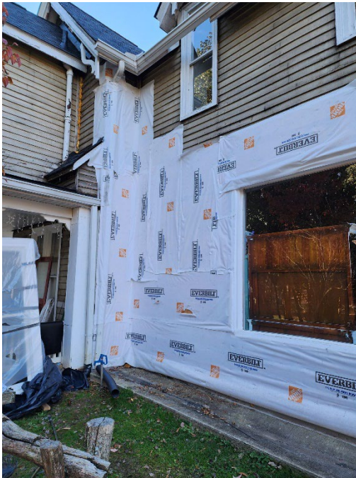
Inside corner with water filtration problem
